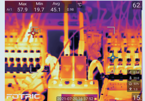
Inverter and Junction Box Monitoring
